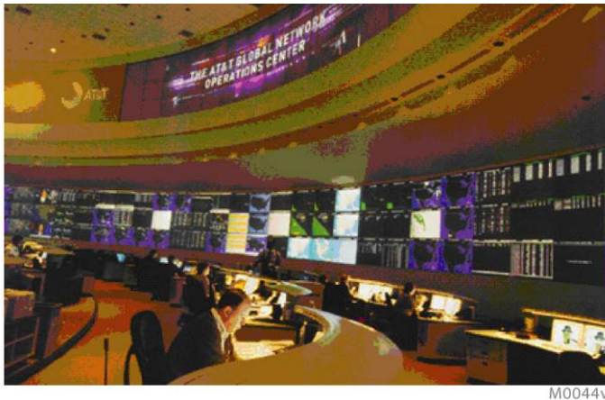
Figure 2.3.1-1: AT&T's GNOC Global Wall Display. AT&T uses the largest and most sophisticated command-and-control center of its kind in the world to service Networx.
