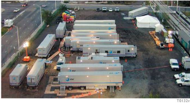
Figure 5.0.3-1: AT&T's Response to World Trade Center Disaster. Equipment and personnel can be en route to an emergency incident within two hours of an official call-out.
