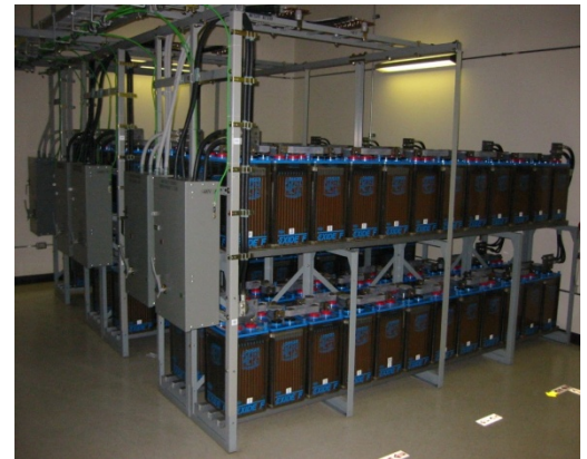
Figure 3: Backup Power Supply
